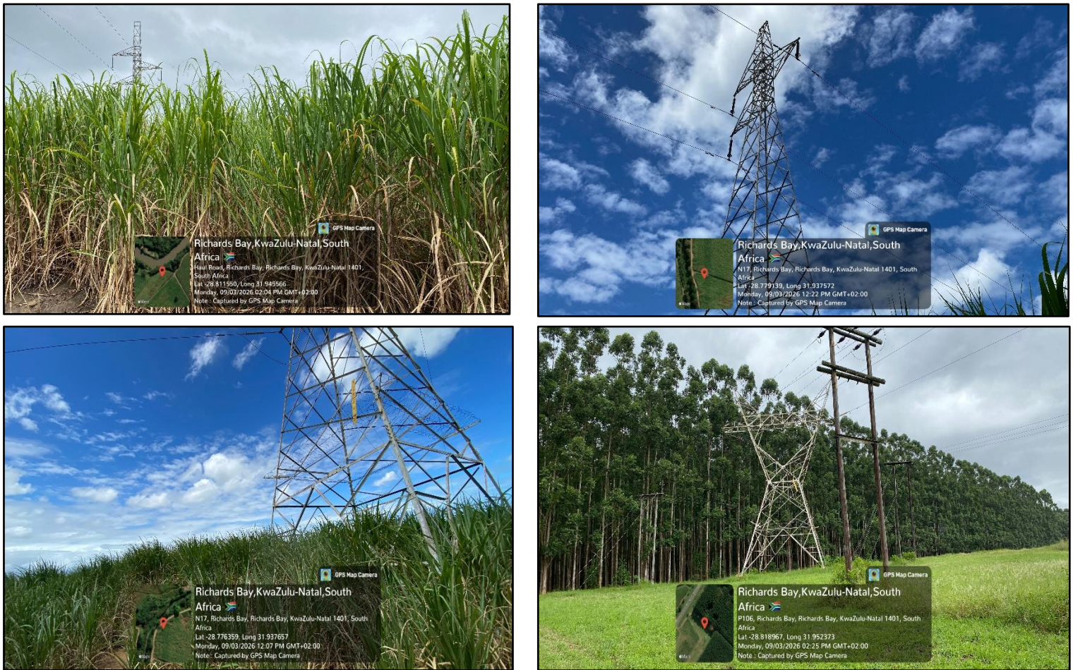
Figure 3: Pictorial Evidence of Photographic records of the existing powerlines with some corroded pylons
